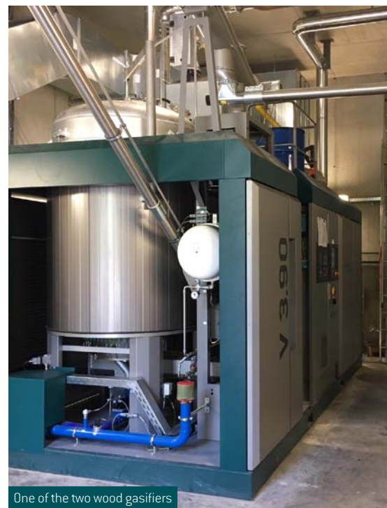
Because of limited space, the CHP is on a higher level.
